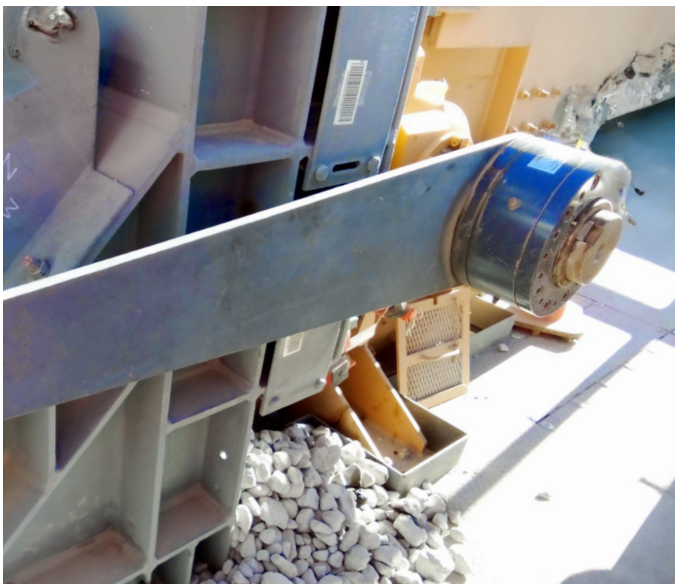
Low Speed Backstop FRHD with special torque arm in Incline Conveyor
