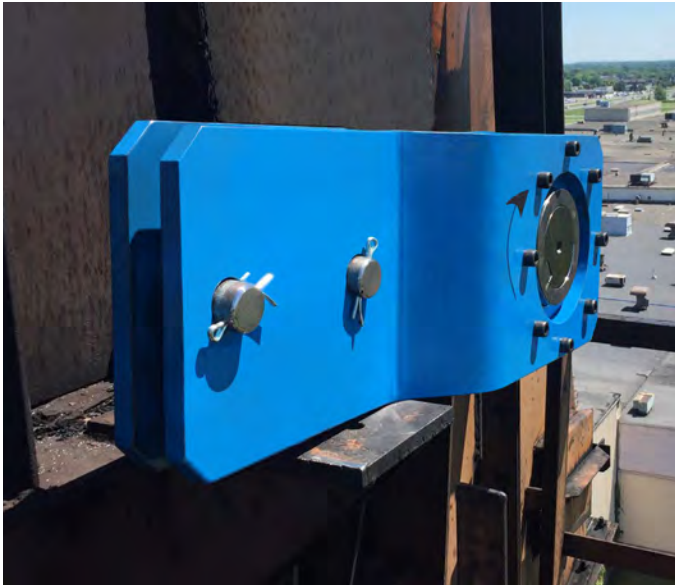
Low Speed Backstop FRHD 900 in Incline Conveyor
