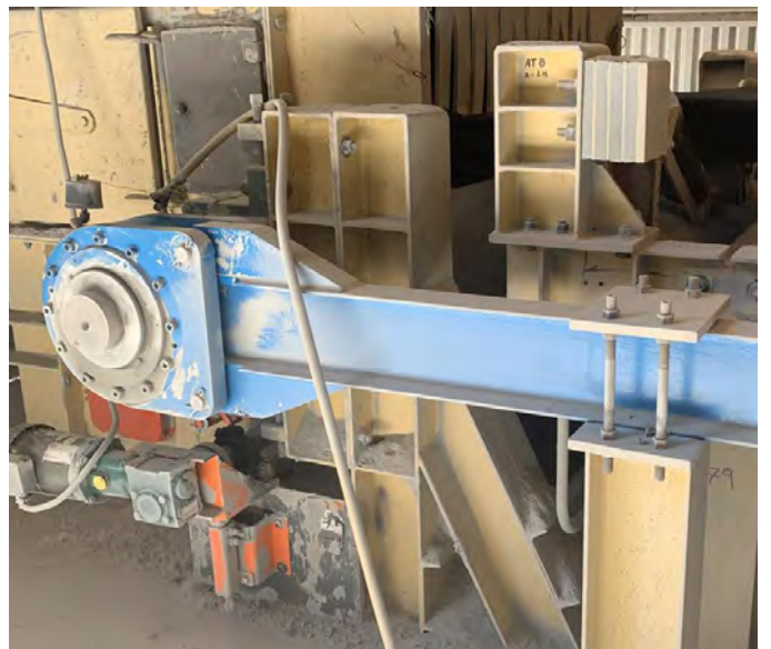
Low Speed Backstop FRHD 1400 in Incline Conveyor
