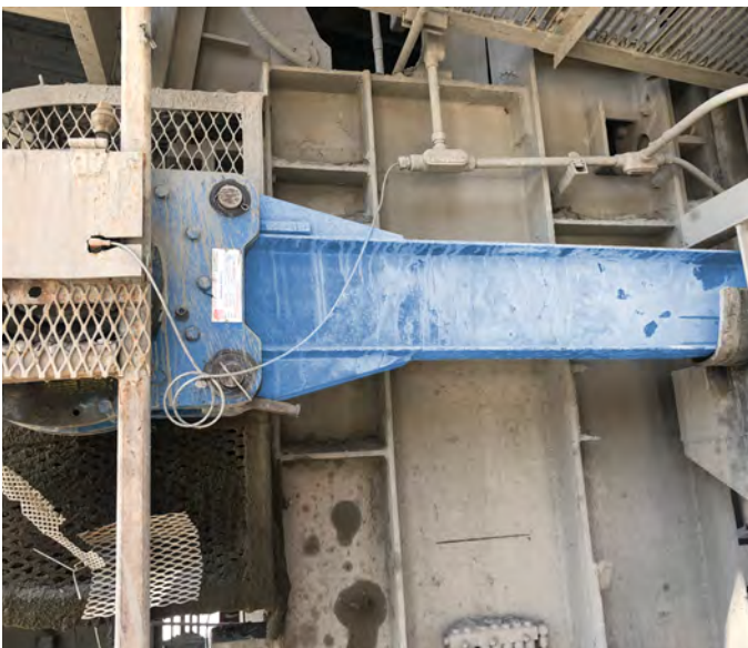
Low Speed Backstop FRHD 1450 in Incline Conveyor
