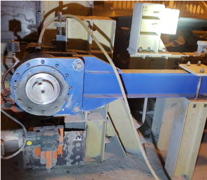
Low Speed Backstop FRHD 1400 in Incline Conveyor
