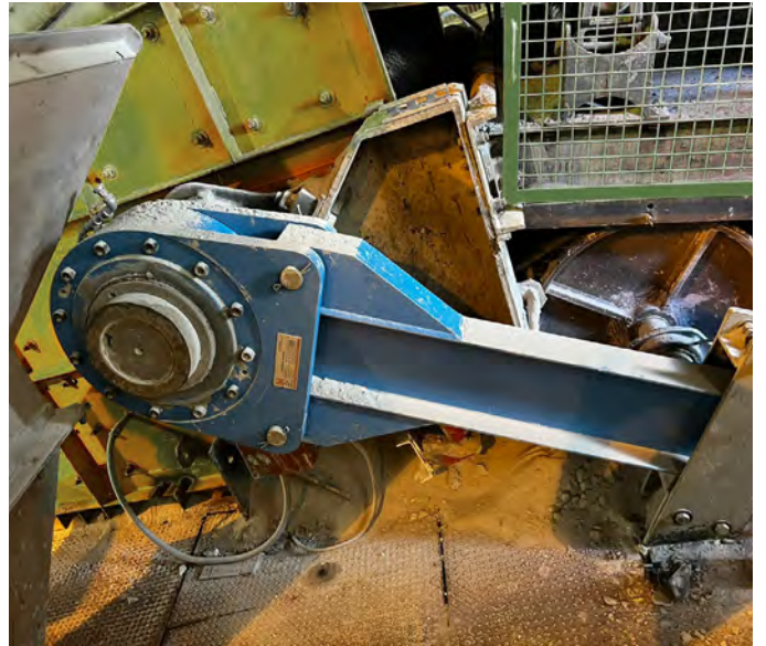
Low Speed Backstop FRHD 1500 in Incline Conveyor
