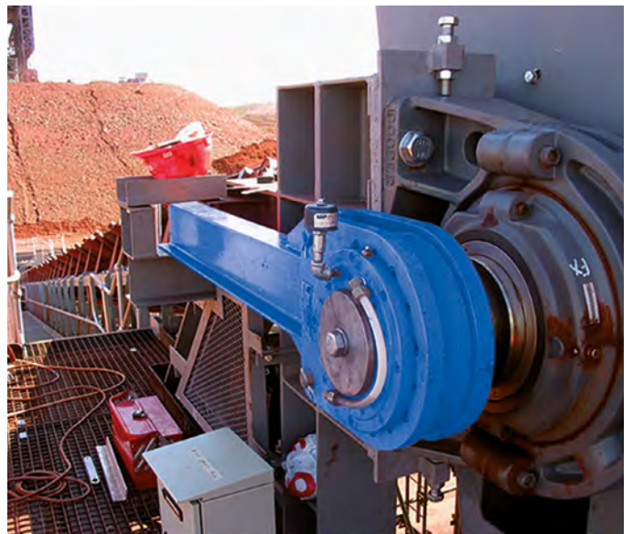
Low Speed Backstop FRHD 1700 in Incline Conveyor
