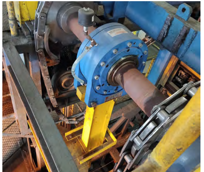
Low Speed Backstop FRHD 1200 in Incline Conveyor
