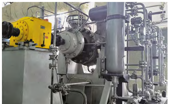
Housing Freewheel FH 4000 in recovery steam turbine
